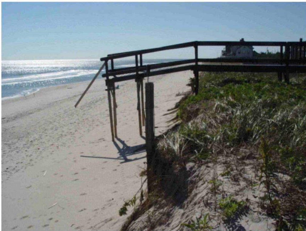
Photoplate 3b. By October 17, 2005 a pair of mild northeast storms had re-excavated the seaward dune slope sweeping away the snow fence at the dune toe and partially destroying the stairs. Note that the erosion went exactly as far as it had two years earlier. Sand was moved into place once again in the spring of 2006.
