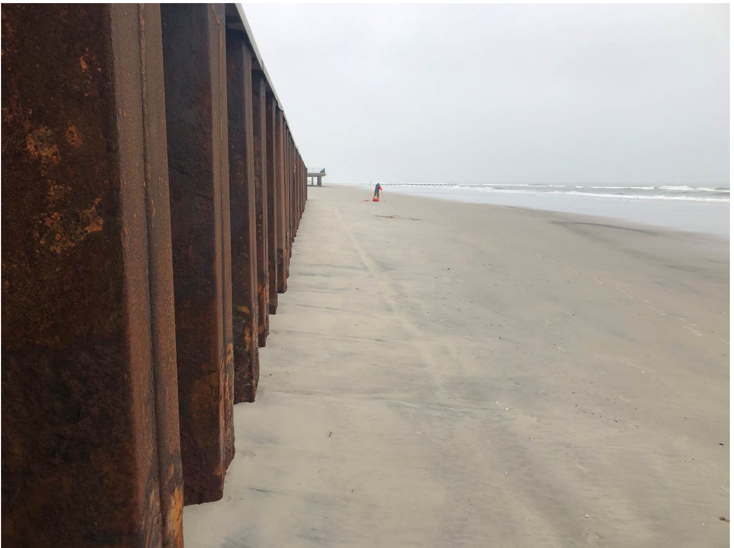
Figure 23. View to the north taken on October 28, 2019 near 26 th Avenue showing the beach at the Surfside Pier's seaward end steel bulkhead. Waves easily reach the bulkhead making a dry berm unlikely until the shoreline advances about 100 feet further seaward. Little change has occurred at the bulkhead in over a year with summer accumulations allowing minor beach use immediately seaward of the steel wall.
