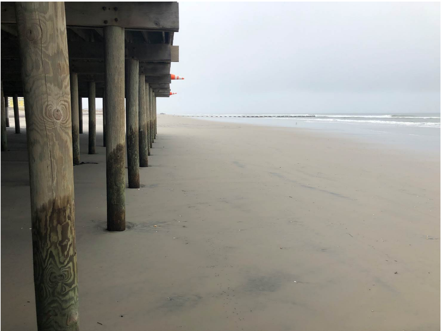
Figure 20. The northern timber pier lies in the surf zone after shoreline retreat. The flat beach is wide and would accumulate sand if it were available to move onto the shoreline. This view was taken October 30, 2019.
